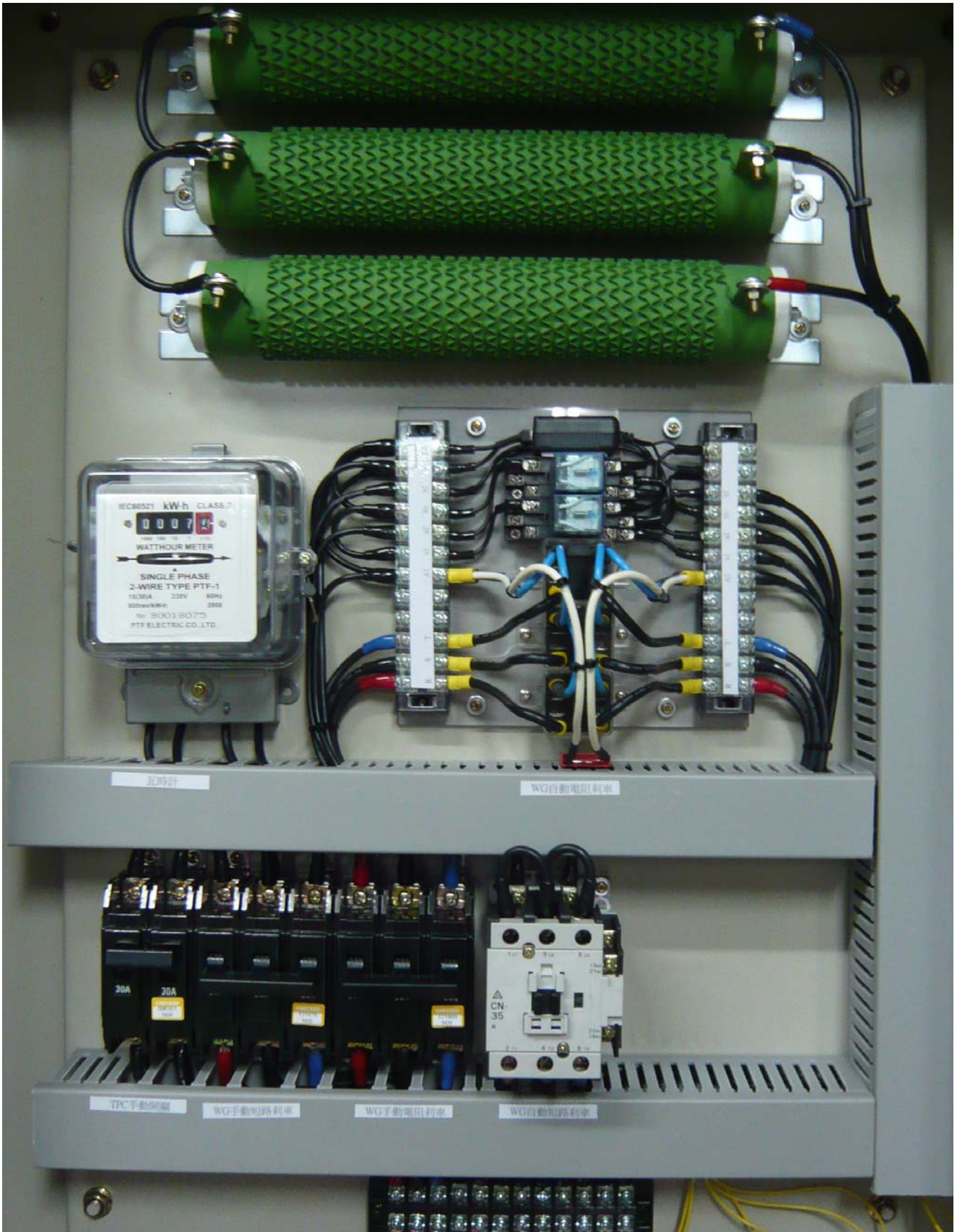
Figure 9 Brake Control Cabinet Placement
